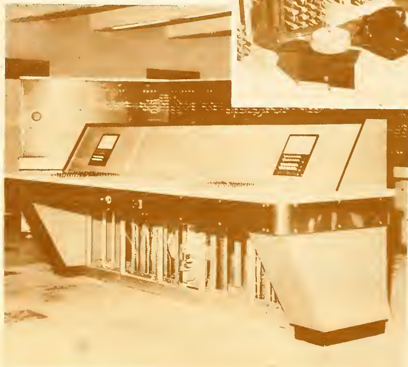
Painéis de Controle — CTC — EFSJ
