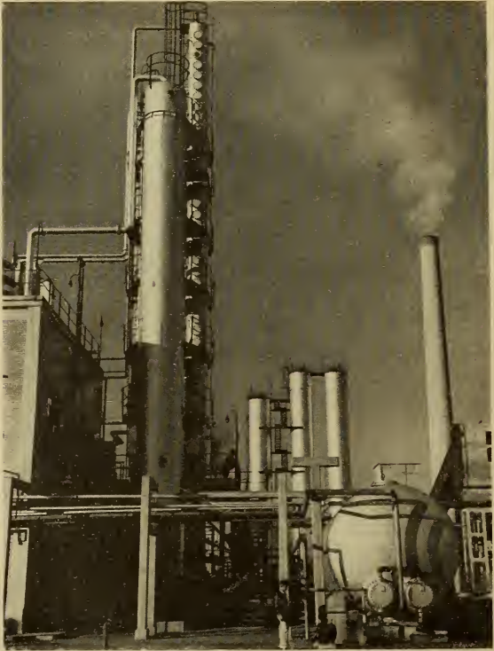
Plant for recovering ammonia, benzene and other by-products from coke-oven gas of Volta Redonda
